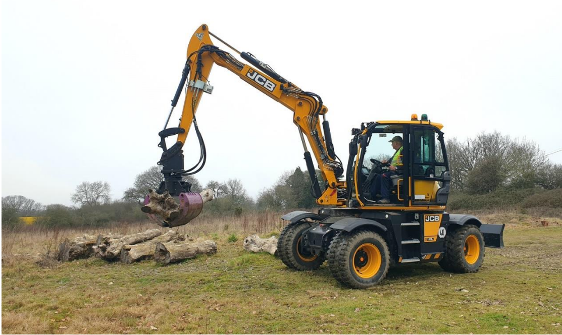
Figure 51- Gatwick Construction JCB assist with moving large deadwood to create habitat piles at the edges of Rolls Field. February 2023 © Rachel Bicker
